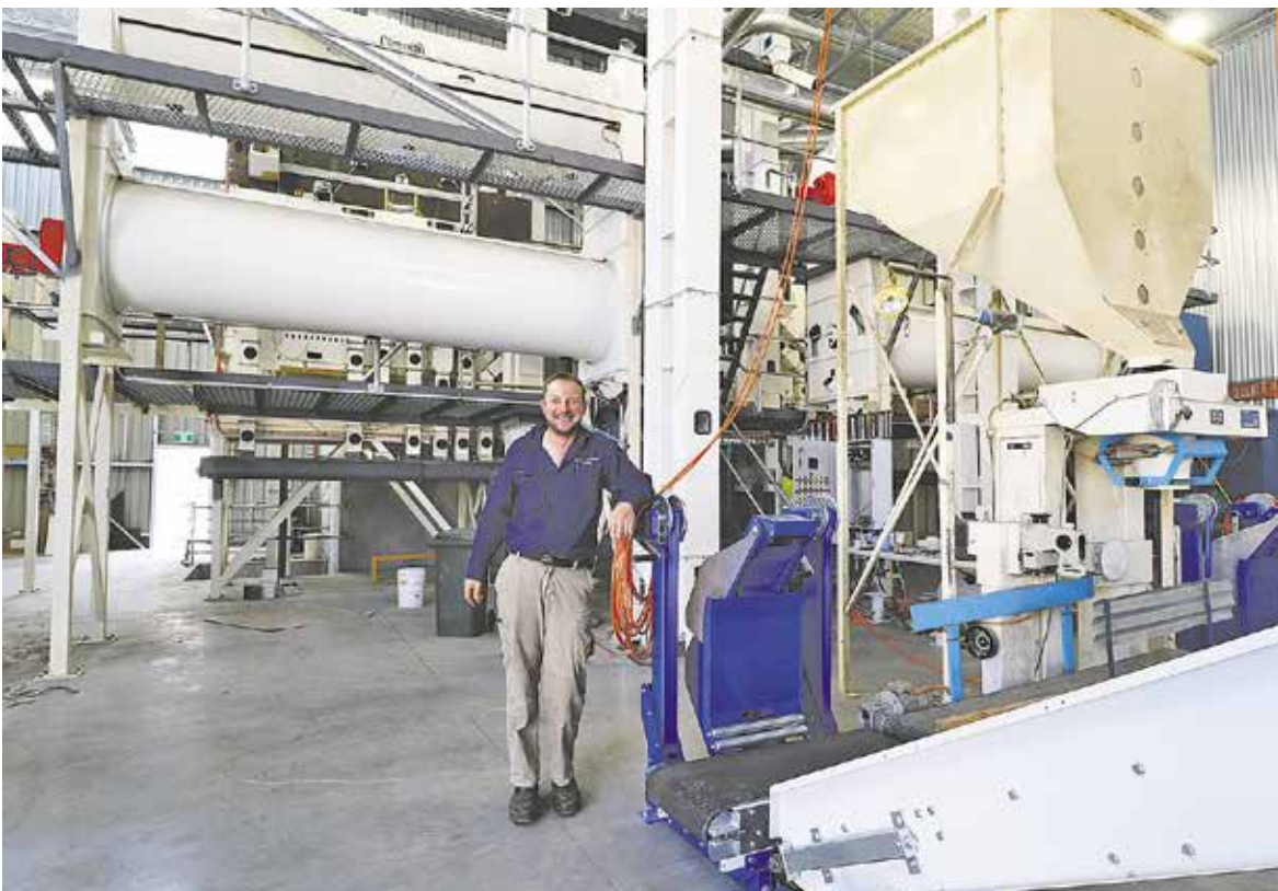
Duncan stands in front of the new seed cleaning machines and beside the new bag stacking facility
