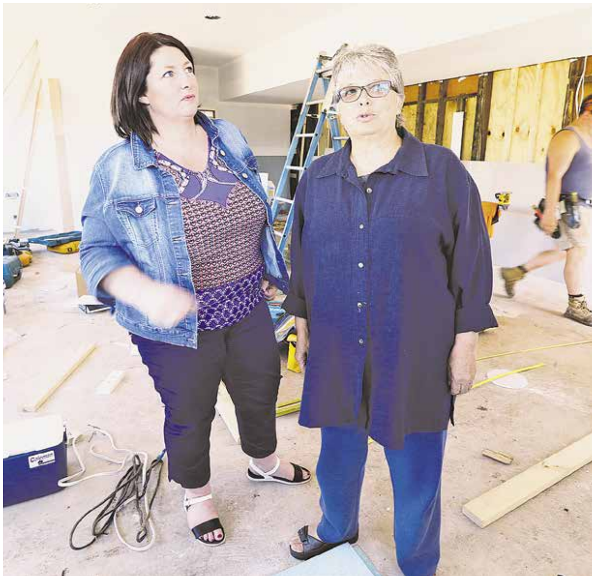
Narelle Whatley and Ros Albiston survey the extension under construction at Deloraine House
