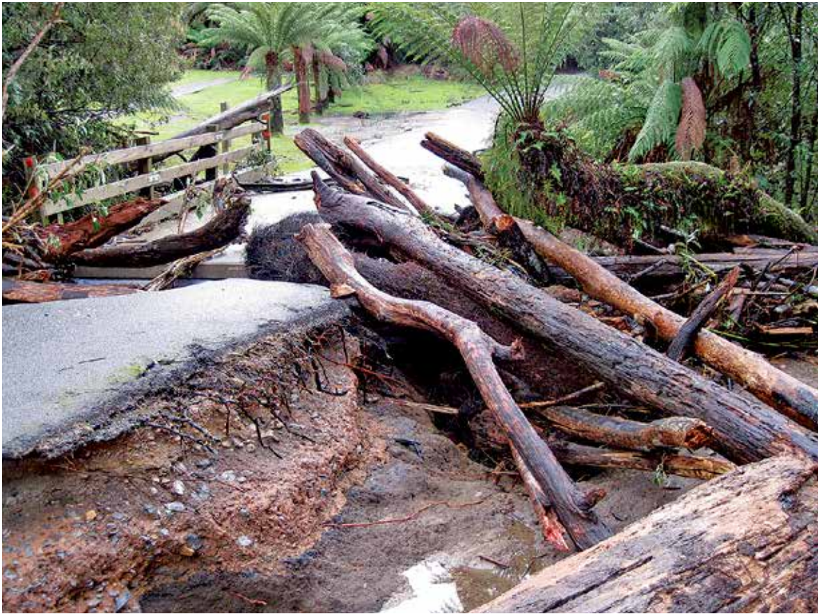
Extensive damage to the road leading to Marakoopa Cave. Photo courtesy of Tas Parks & Wildlife
