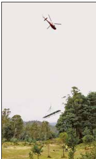
A chopper lifts the Liffey foot bridge into place in order to reopen a popular Falls track.
