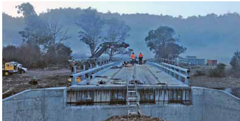
The much-awaited Liena bridge replacement is gradually nearing completion. Pictured above, workmen prepare to put the final sections in place. Photo by: Todd Wilson
