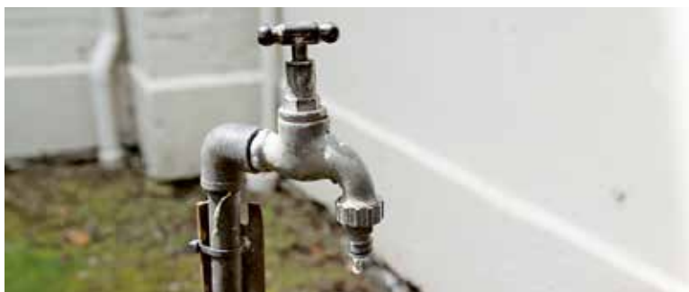
A slow dripping tap can waste up to five litres of water per hour.
