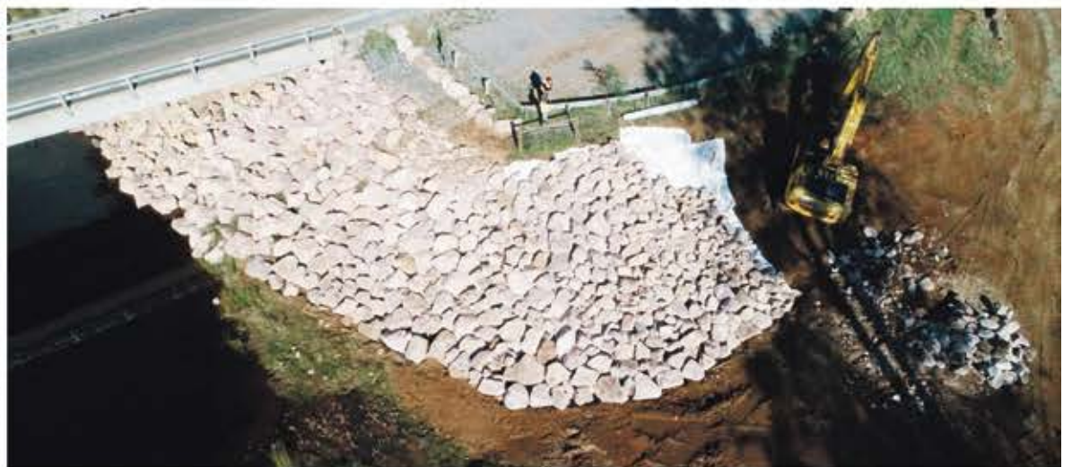
Above: Aerial image of the additional embankment protection work just prior to completion
