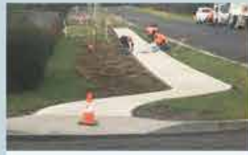
Footpath Construction Moriarty Street Deloraine from Stagg Court to Tower Hill Street
