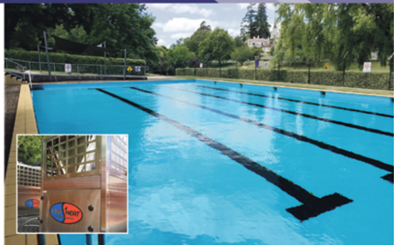
Above: Deloraine Swimming Pool now a constant 24 degrees due to the new pumped heating system (inset)
