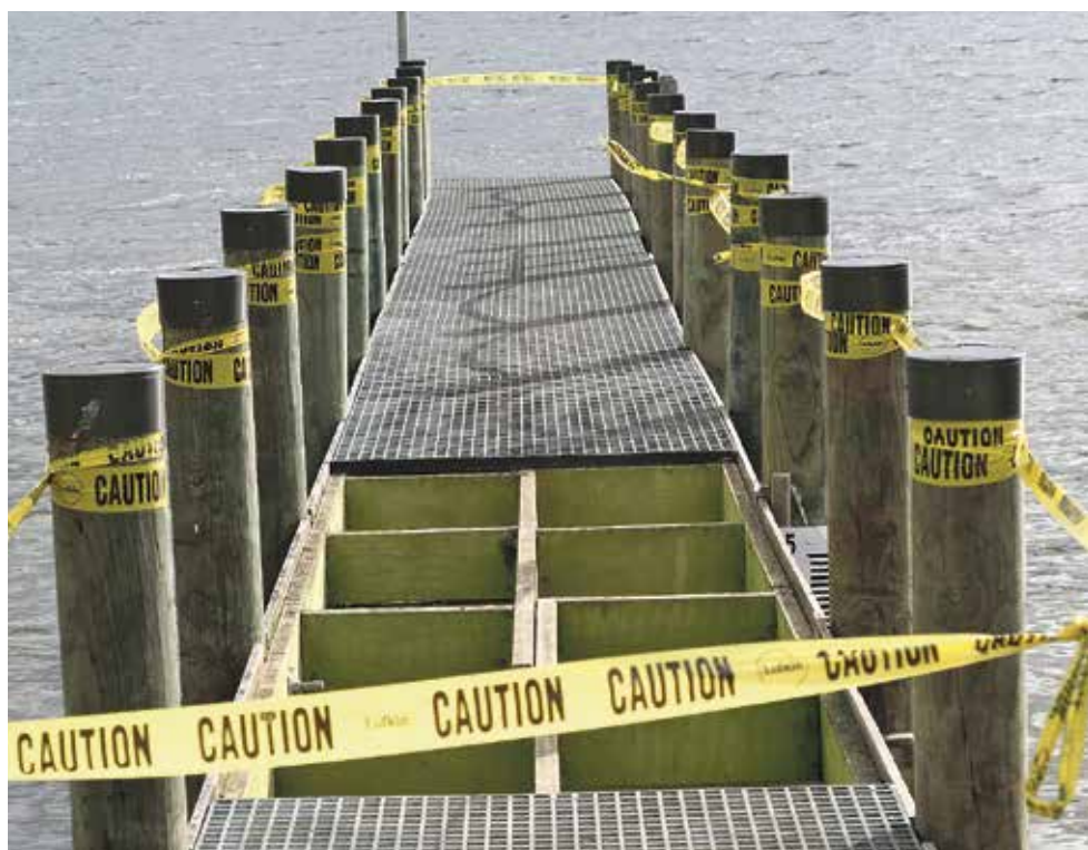
Metal grating from Four Springs jetty was stolen recently, making the jetty temporarily unusable. Photo supplied
