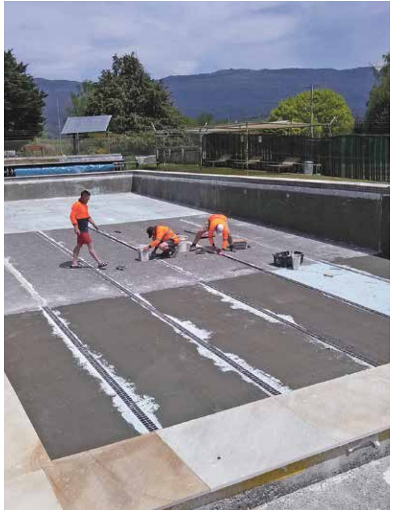
Mole Creek swimming pool is scheduled to reopen in the new year, after leaks were plugged and joints repaired, courtesy of a grant from the Tasmanian Community Fund. Photo supplied
